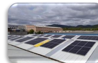
Sentmenat (2023) Members: 4 (industrial) Power: 40 kWn
